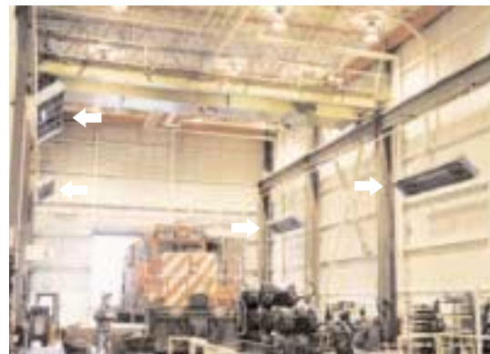
Canadian Pacific Railroad Diesel Repair Shop heated with 8 RSTP17's mounted 20' above finished floor.
